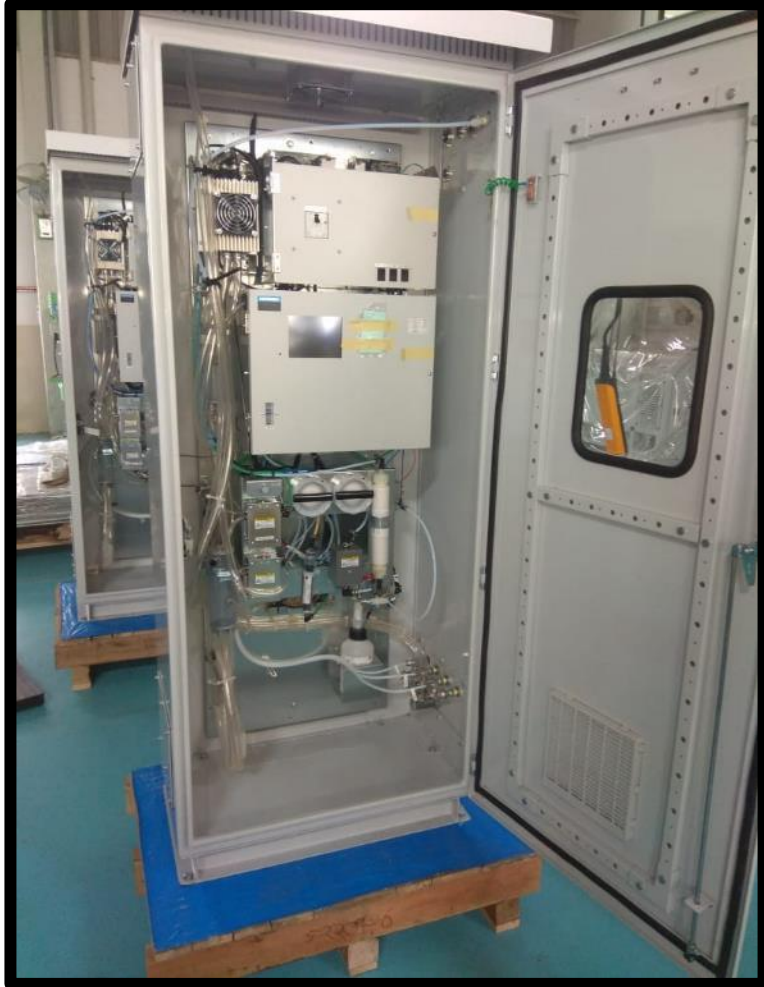
Well Engineered Japanese Systems for CEMS Application.
